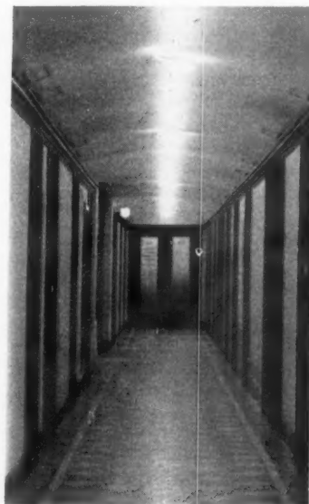
Neon tubes now supply lighting for the corridors of the Majestic building since an air conditioning installation made it necessary to install false ceilings in all hallways. Conventional lighting fixtures would have projected too far downward.
